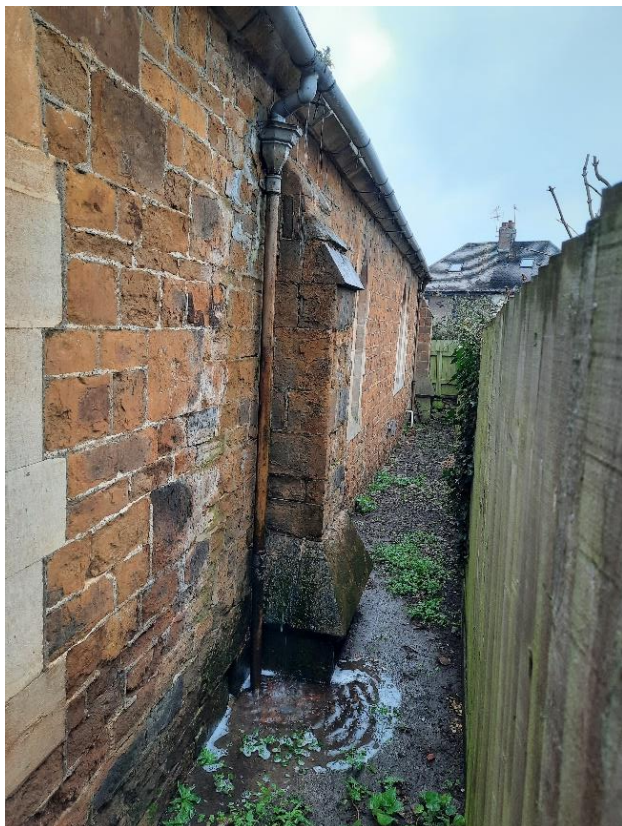
Figure 1: Overflowing gutters and a non-functioning drains
