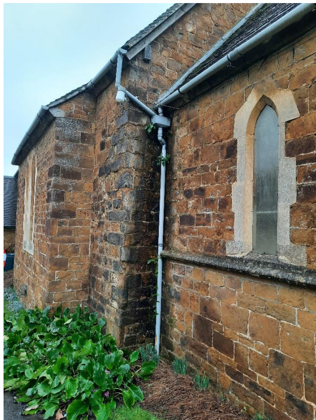
Figure 2: Badly maintained downpipes have led to saturated walls with plants growing out of them...
